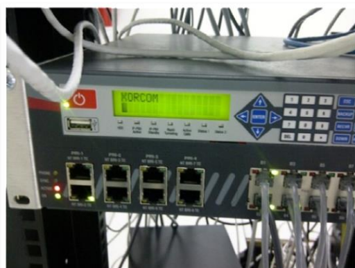
Xorcom XE3000 installed at TBC Ball factory
